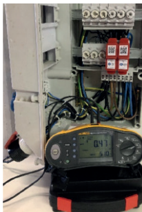
Loop impedance measurement on a sub-distribution with CEE 16 adapter, measured with a test device according to DIN EN 61557-3 (VDE0413-3), (can be used independently of the manufacturer)
