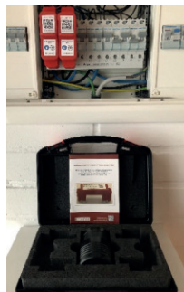
RCD test adapter in the sub-distributor for loop impedance measurement
