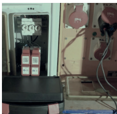
Loop impedance measurement on a site power distributor with CEE 16 adapter
